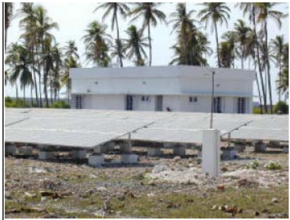
Fig.2. 100 kW SPV Installation at Kavaratti Island
